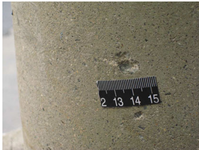
FIG. 2—The ovoid 1.1- by 1.1-cm hole on the concrete telegraph pole at the scene.
